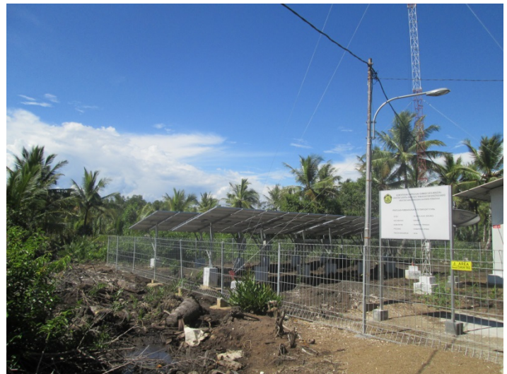
PV system built for the government to power a village
