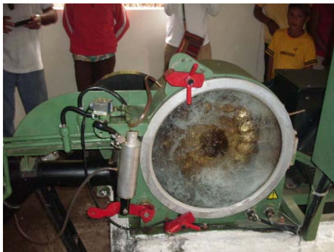
Examining the Pelton wheel generator
